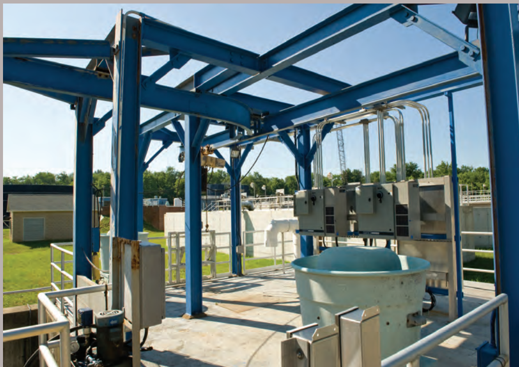
The pump station at MAWSA.
