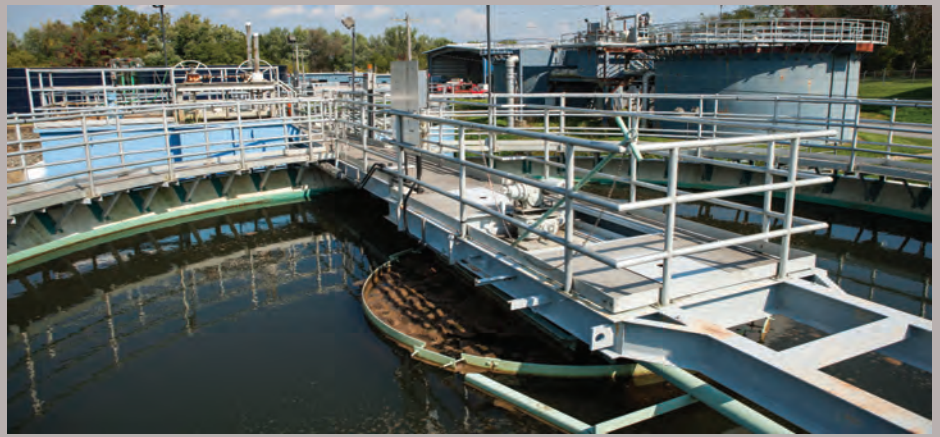
A section of the oxidation ditch at MAWSA.
